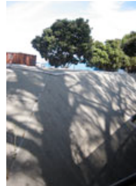
Berm used to contain hazardous wastes Photo: Steve Lerner
